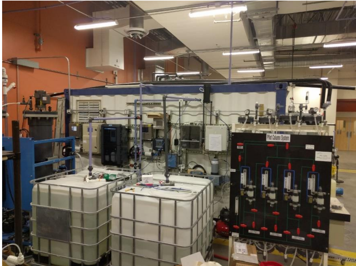
< 4-inch column activated carbon system >
